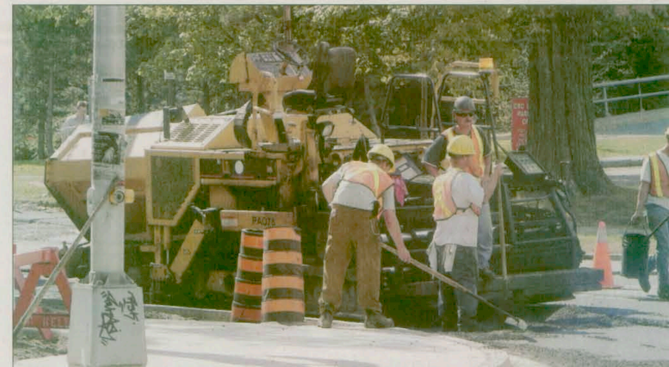
Road workers add new asphalt to a section of Summer Street in Halifax.
