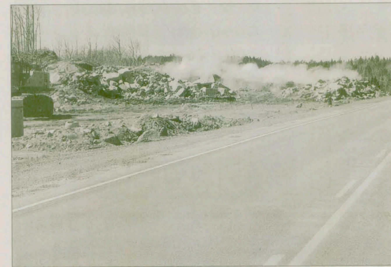
Rock excavation becomes more expensive and takes more time because the additional cost of blasting must be considered, as well as restrictions on the size of blasting that can be done at one time, and the times of day when you're allowed to do it.
