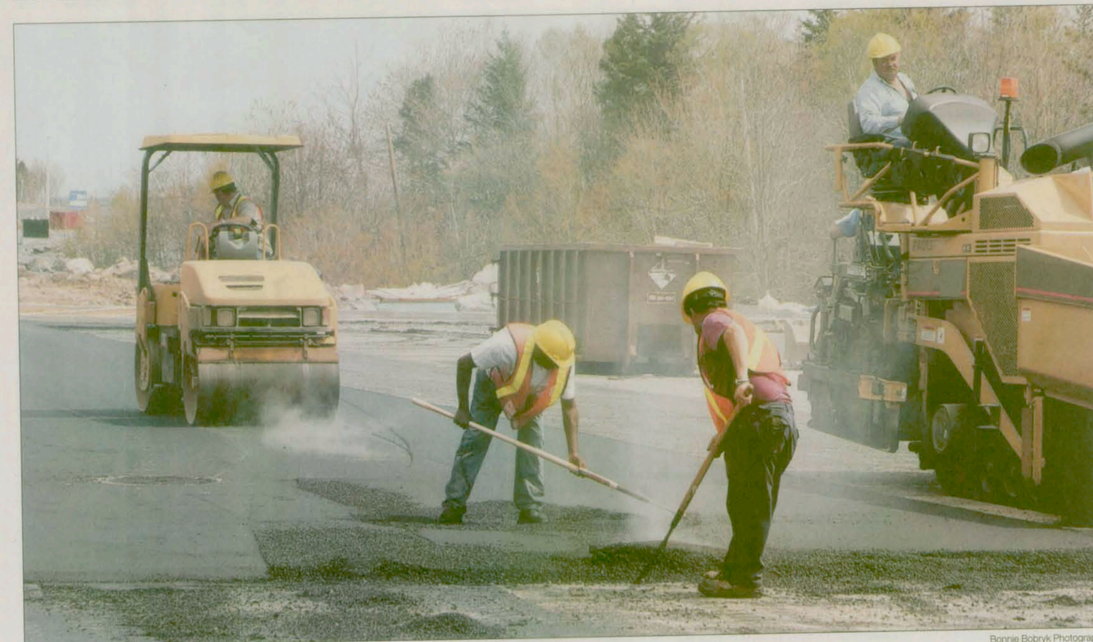
Road work continues on one of the largest ongoing retail construction projects east of Calgary at Dartmouth Crossing.
