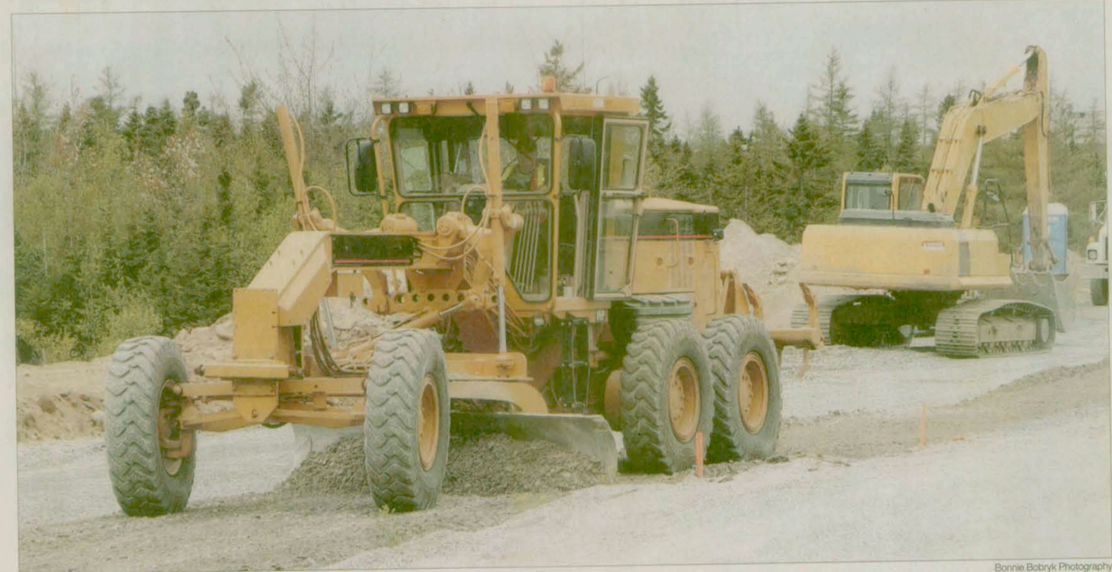
While road building has a long and storied history in Nova Scotia, going back more than 100 years, today it's one of the province's most modern and progressive sectors. Road builders work on the Commodore Drive extension in Burnside Industrial Park in Dartmouth May 28.
