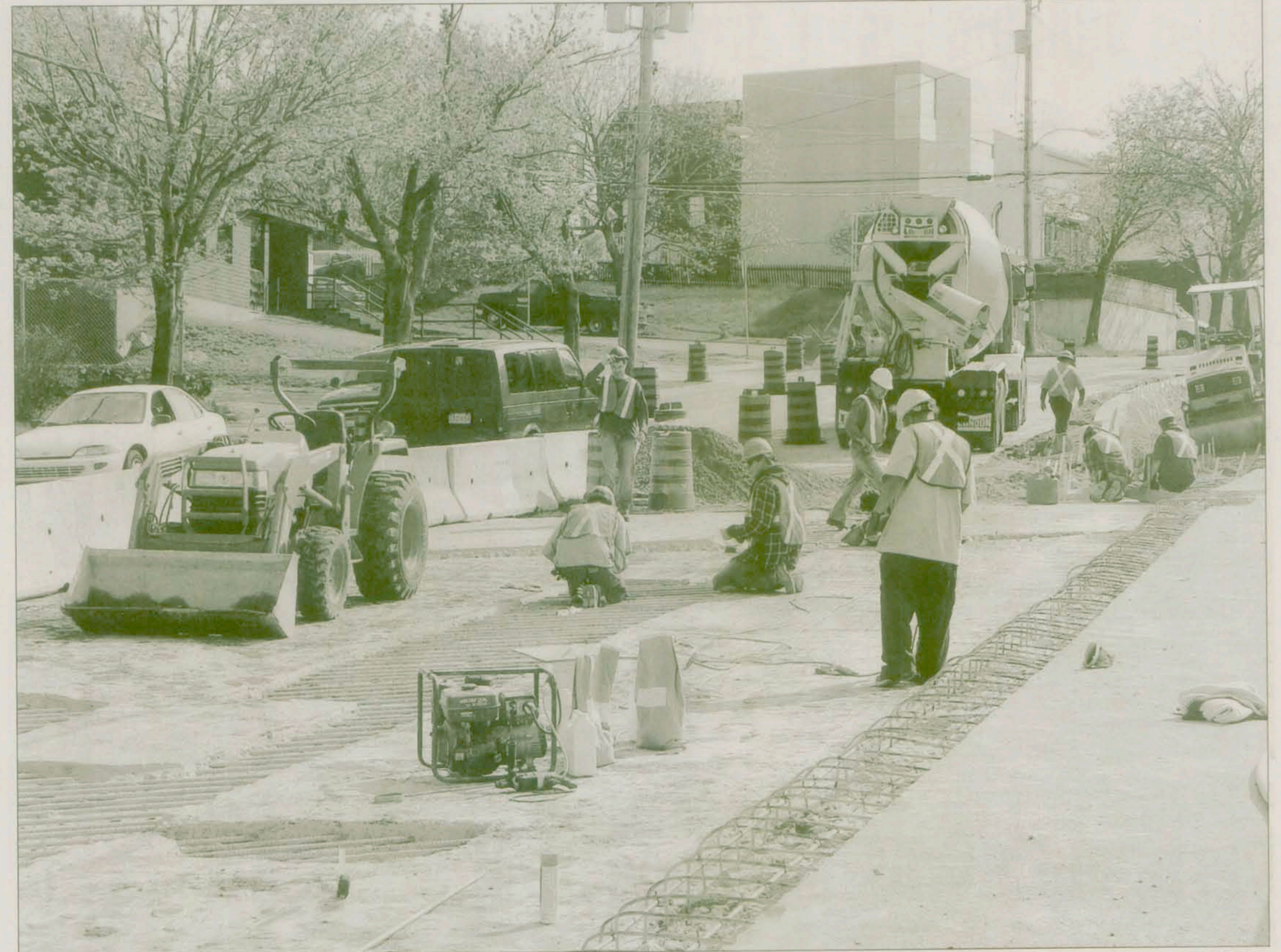
The road-building industry in Nova Scotia employs 7,500 people and pays an estimated $375 million in wages annually. Its payroll and benefits far exceed minimum standards. Hourly rates for many road building jobs range from $13 to $22 per hour. Workers prepare an overpass, above, on Lady Hammond Drive in North End Halifax recently for concrete resurfacing.
