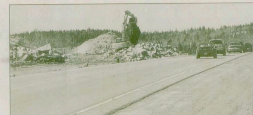
The excavation of materials is the most costly and time-consuming process in road construction here in Nova Scotia.
